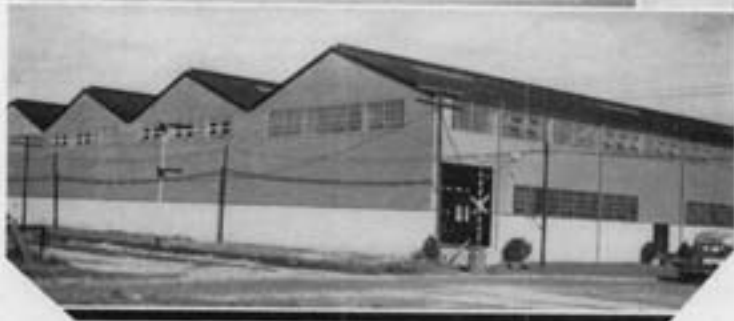
TOP: Office of the Bethlehem Steel Company. BOTTOM: Part of Bethlehem's Steel Warehouse, under construction.
