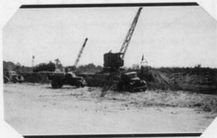
Extension of Wingate Street to make way for new Appraisal Stores Building.
